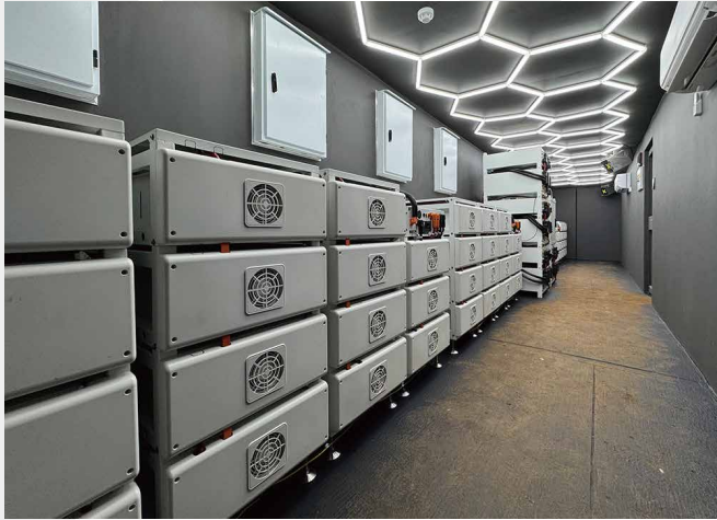
South Africa ▶ Model: 125kW PCS*4 + MPPT*4 + 500kW STS*1 Battery: BOS-B*4 Capacity: 500kW/860kWh
