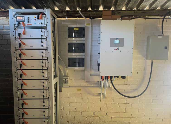
South Africa ▶ Inverter: SUN-50K-SG Battery: BOS-G Capacity: 50kW/55kWh
